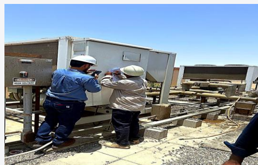
Site Inspection — Rooftop Chiller Unit Technical team recording equipment data on site
