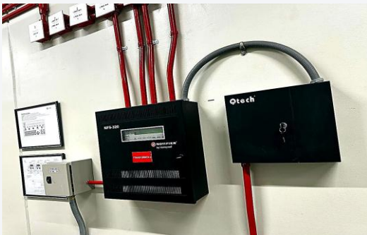
Fire Alarm Control Panel (FACP) Fire detection and notification panel
