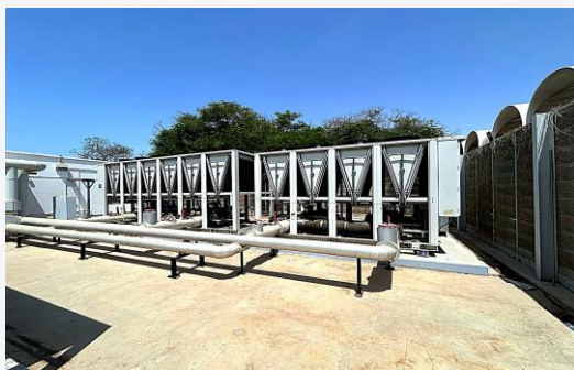
Chiller Plant — Rooftop Bank Multi-unit chiller bank with header piping
