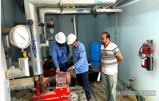
Site Inspection — CHW Pump Room Technical team reviewing pump and CHWS piping
