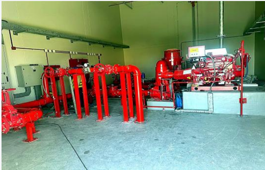
Fire Pump Room Electric and diesel fire pump sets with pipework
