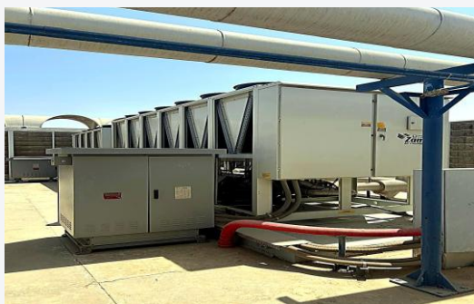
Chiller Unit — Zamil Air Conditioning Control panel, piping, and flexible connections
