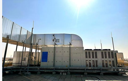
Rooftop AHU & Chiller Installation Package AHU, ductwork, and chiller plant
