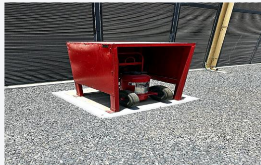
Fire Hose Reel & Extinguisher Station Mobile hose reel and extinguisher cabinet
